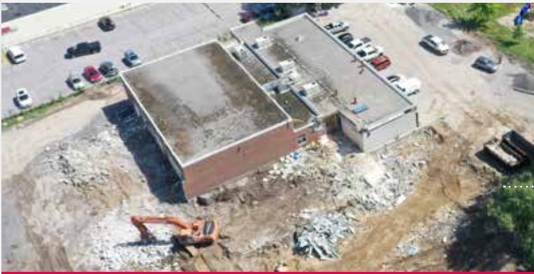
Construction progress underway at the St. Joseph Catholic School site in Belleville.
