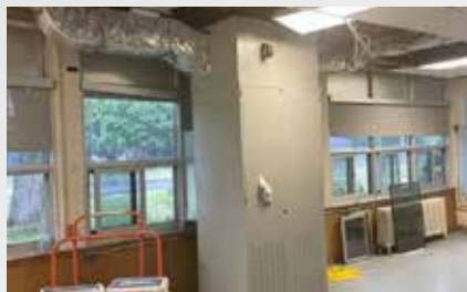
The ALCSDB continues to make the improvement of ventilation systems at our sites a priority by ensuring regular inspection and servicing of our systems. Ventilation upgrades through the use of stand-alone HEPA filtration units and the completion of extensive work will improve and optimize ventilation and air filtration within our schools.
